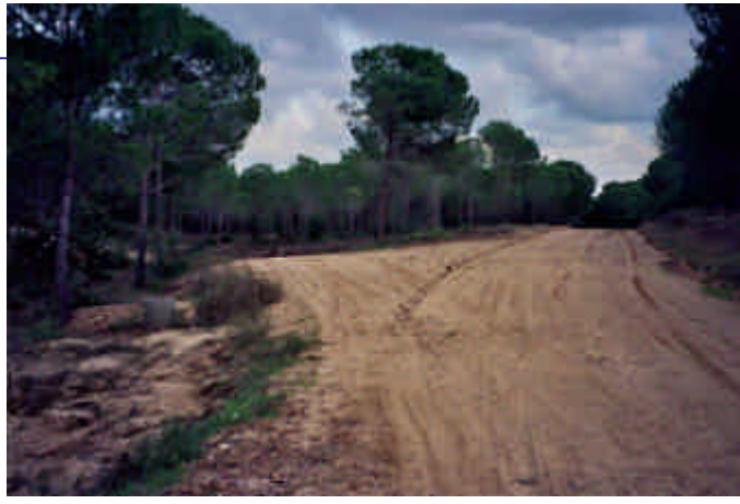
Cutting down of trees, earth moving and flattening operations in the area
